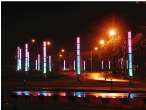
Fig. 1.19. Artistic accent lighting at the main gate of the Science Based Industrial Park located in Hsin Chu, Taiwan (courtesy of K. R. Wang and L.-W. Tu, 2005).
